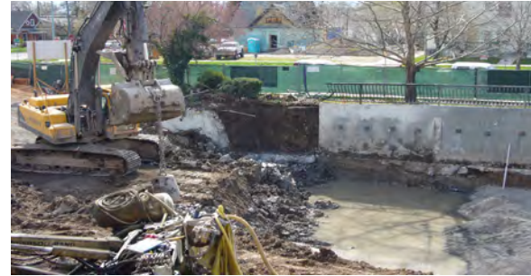
Ground water can have an impact on development. Often times, basements and subterranean parking structures are required to pump ground water to prevent it from damaging buildings.
